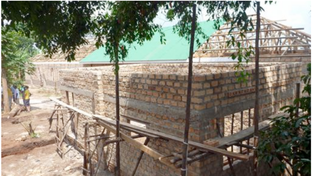
Photograph shows the work completed at the Bukeka Children's Centre towards the end of week 6. Background: the partly roofed multi-purpose building (includes classroom; chicken coop; and store). Foreground: the new school kitchen is built to roof level.
