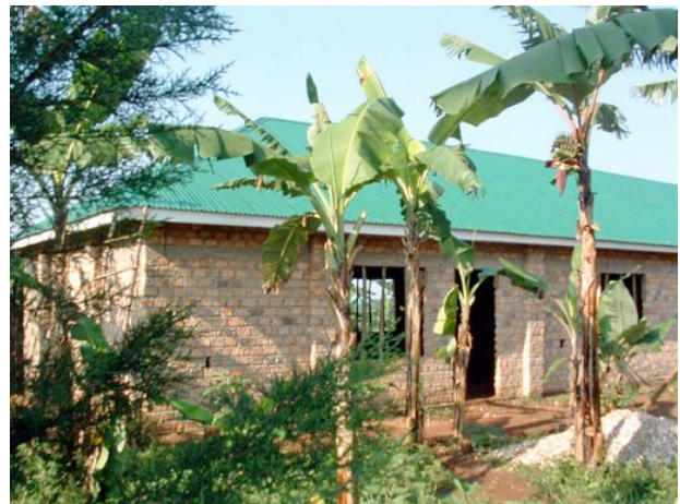
Photograph shows the roofing of the multi-purpose building (Bukeka) has been completed by local builders
